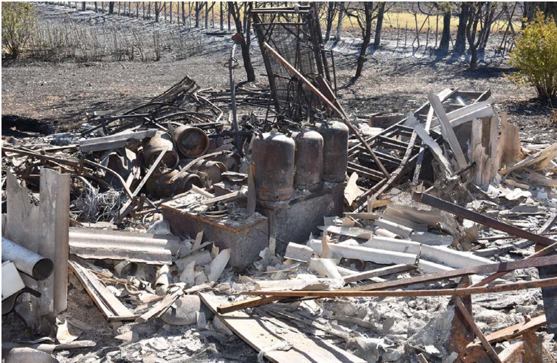
Figure 9. Gas canisters exposed to the combustion of the old house, near the main building.
